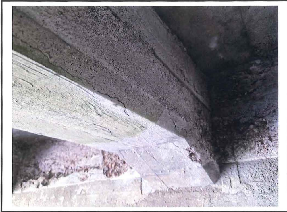
Photo 17 Spall and longitudinal cracks noted on girders
