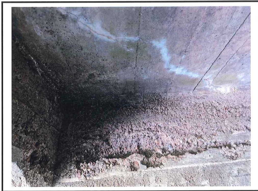
Photo 16 Severe scaling on ballast wall and cracks with efflorescence noted on deck soffit
