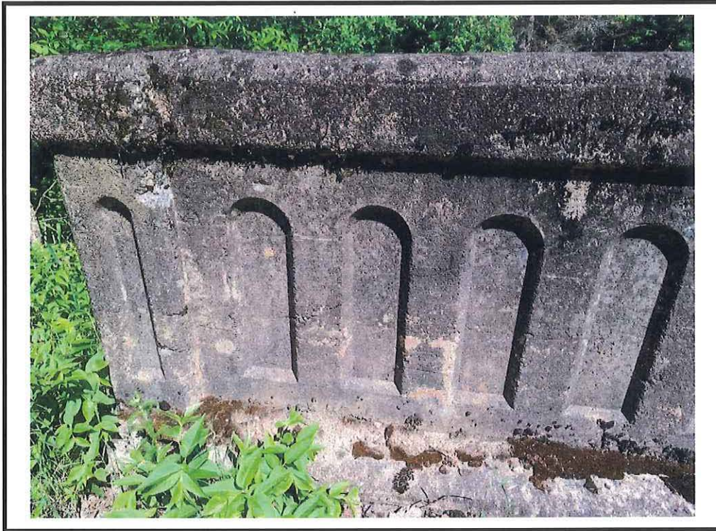
Photo 9 Light to moderate scaling and discoloration noted on parapet wall
