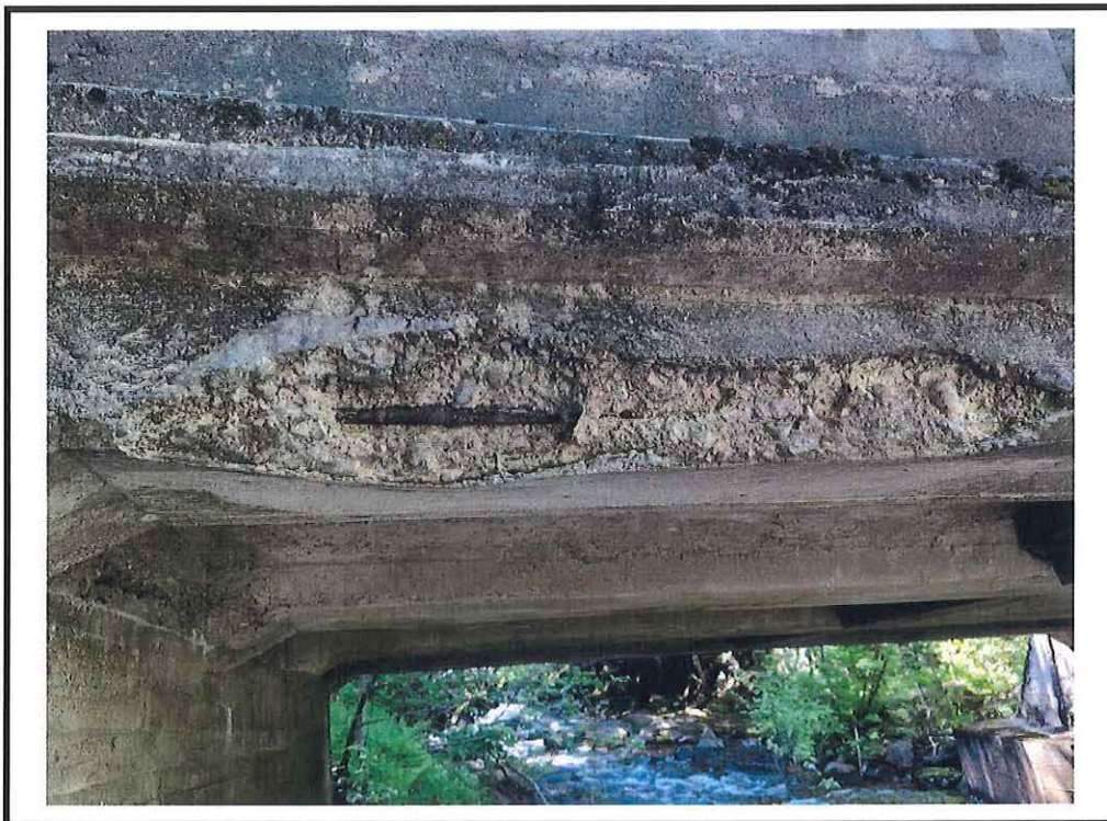
Photo 10 Large spall with exposed corroded reinforcing on north fascia.
