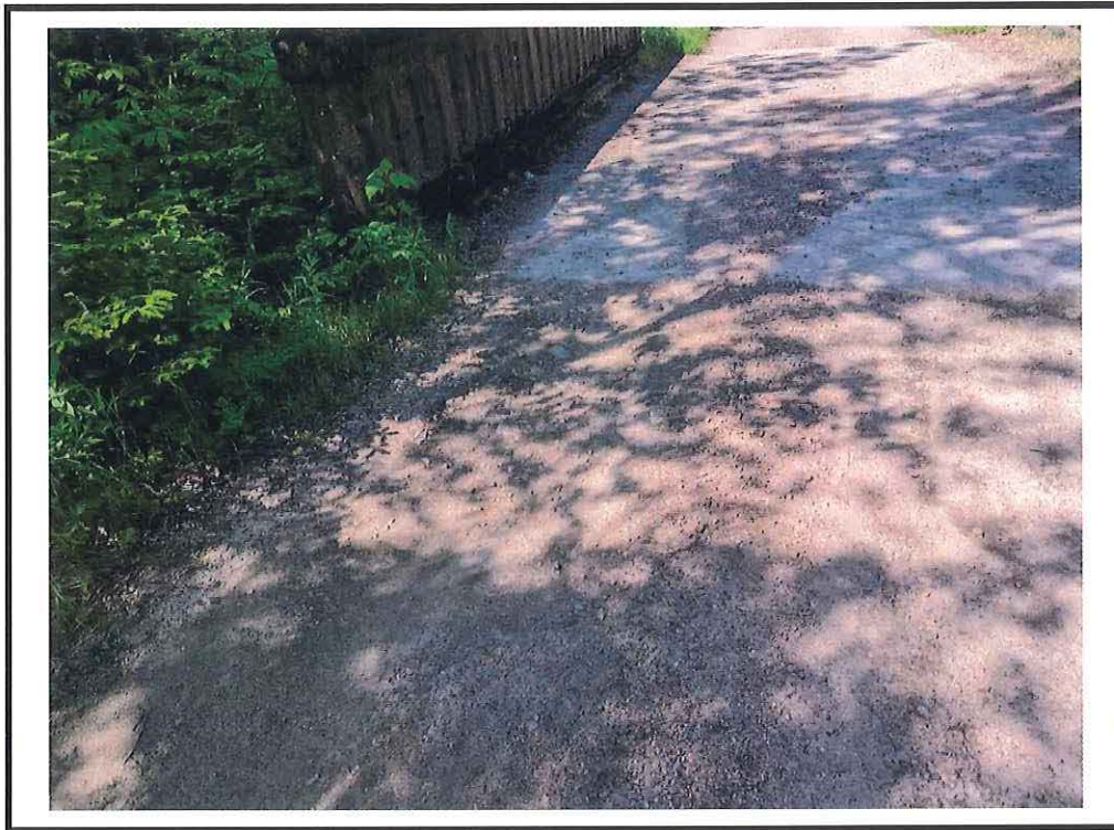
Photo 7 Large potholes on east approach.
